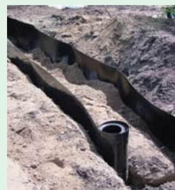
We install our proven barrier 27" deep around the bamboo planting to provide complete and effective containment.
